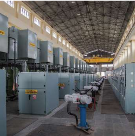
Pump house at Hanamapur, Karnataka
