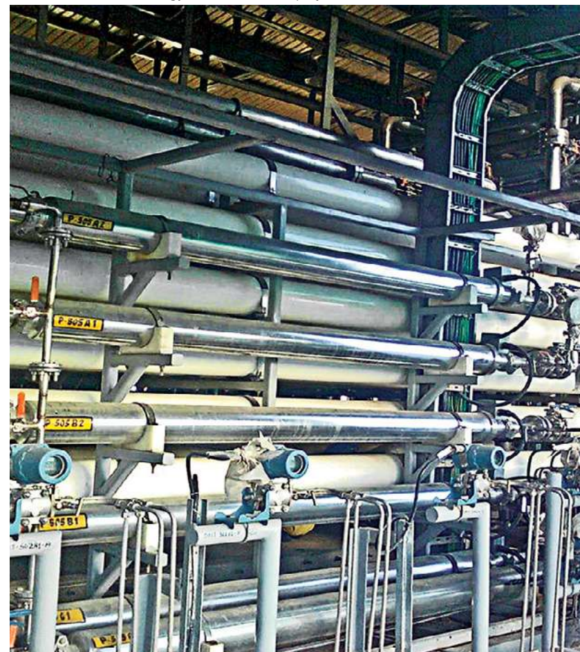
Reverse osmosis technology at a desalination project
