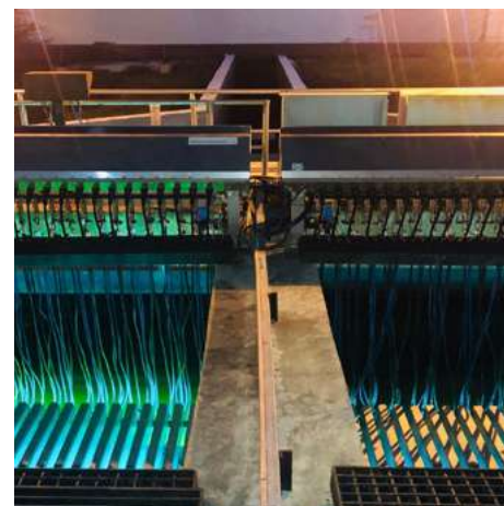
UV Disinfection System
