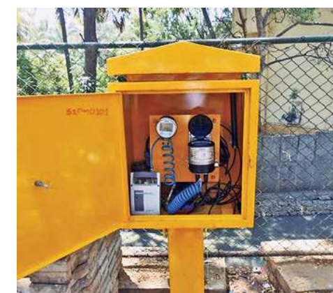
District meter cabinet
