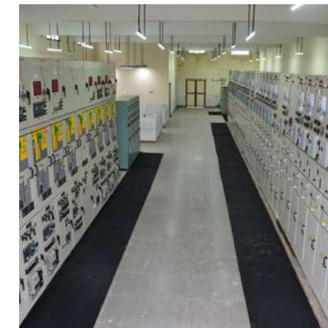
Substation, Bidkin, Maharashtra
