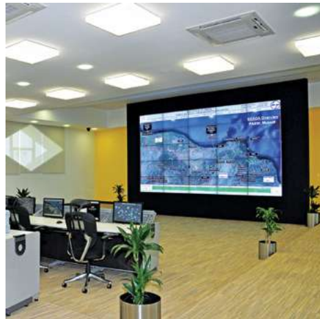
Real-time Project monitoring with SCADA
