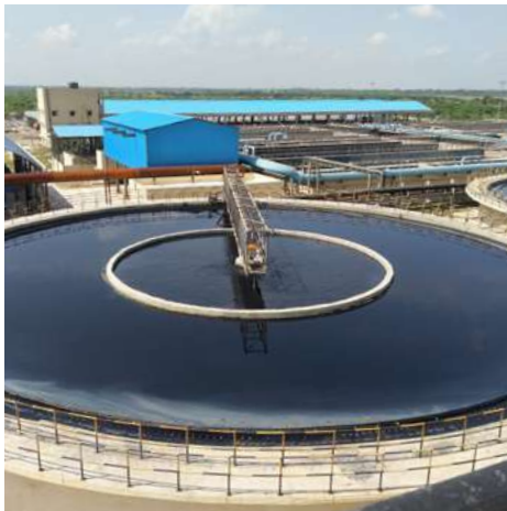
100 MLD Common Effluent Treatment Plant, Narol, Gujarat
