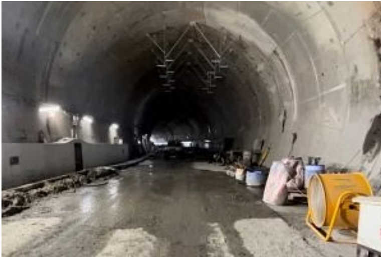
The first of the twin tunnels, which had a breakthrough in 2022 | Manasi Phadke, ThePrint
