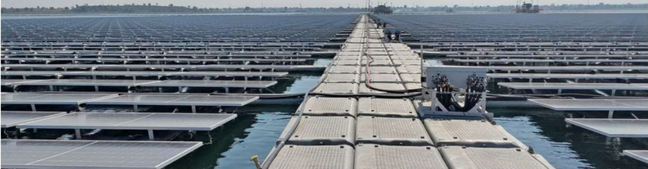
BUOYANT ASSET. The 278 MW floating solar park at Omkareshwar dam on the Narmada in Madhya Pradesh is collectively owned by three entities — SJVN Green Energy, NHDC, and Amp Energy
