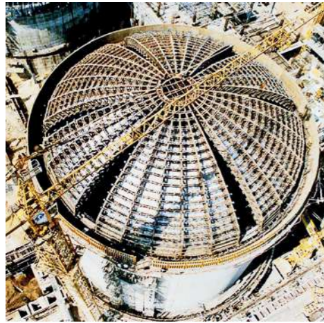
Kaiga atomic power plant
