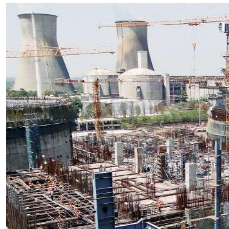
Kakrapar nuclear power plant
