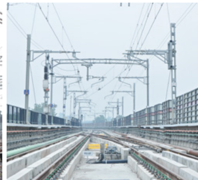
OHE using aluminium single cantilevers in Line 8 - Phase 3 DMRC
