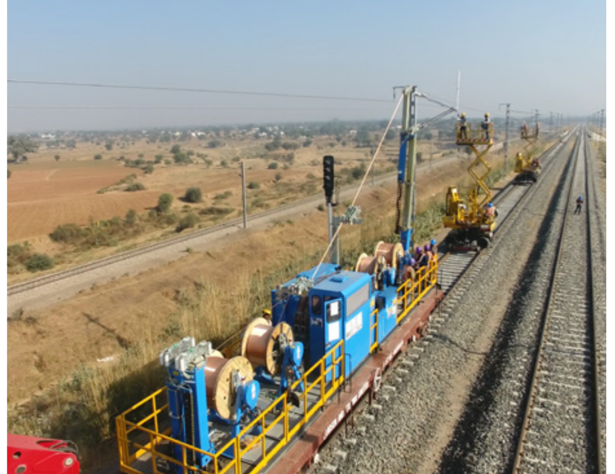
Mechanised Wiring Trains - Enabling high productivity through simultaneous stringing of conductors under tension
