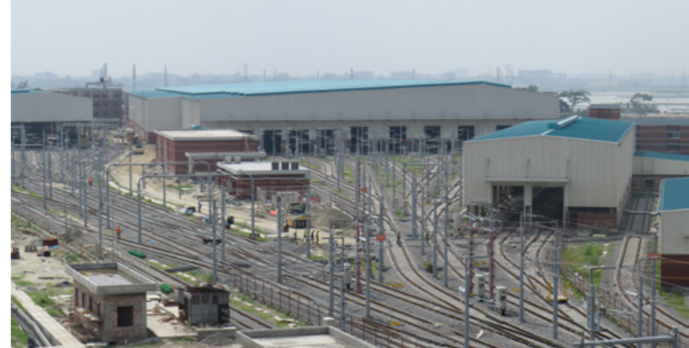
Trackworks and Overhead Catenary System at Uttara Depot
