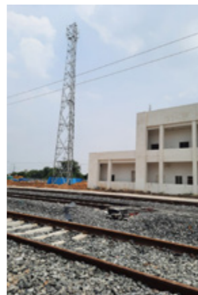
GSM-R tower at CTP14 - WDFC
