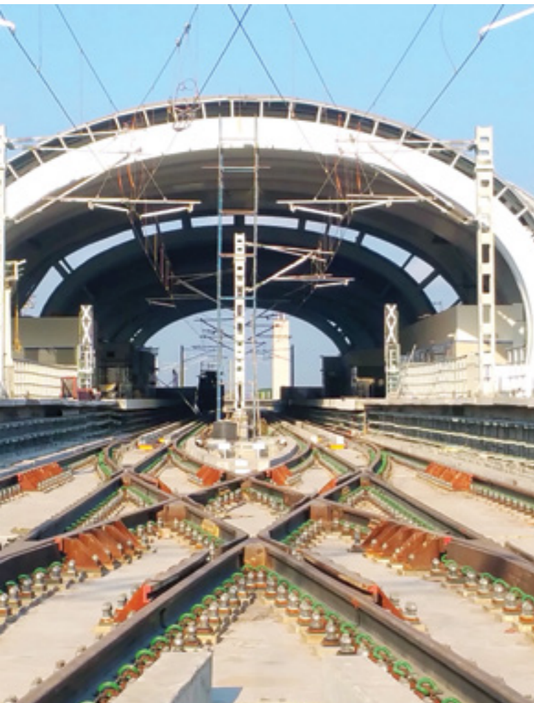
Completed section of Slab Track in a Turnout section of Chennai Metro.
