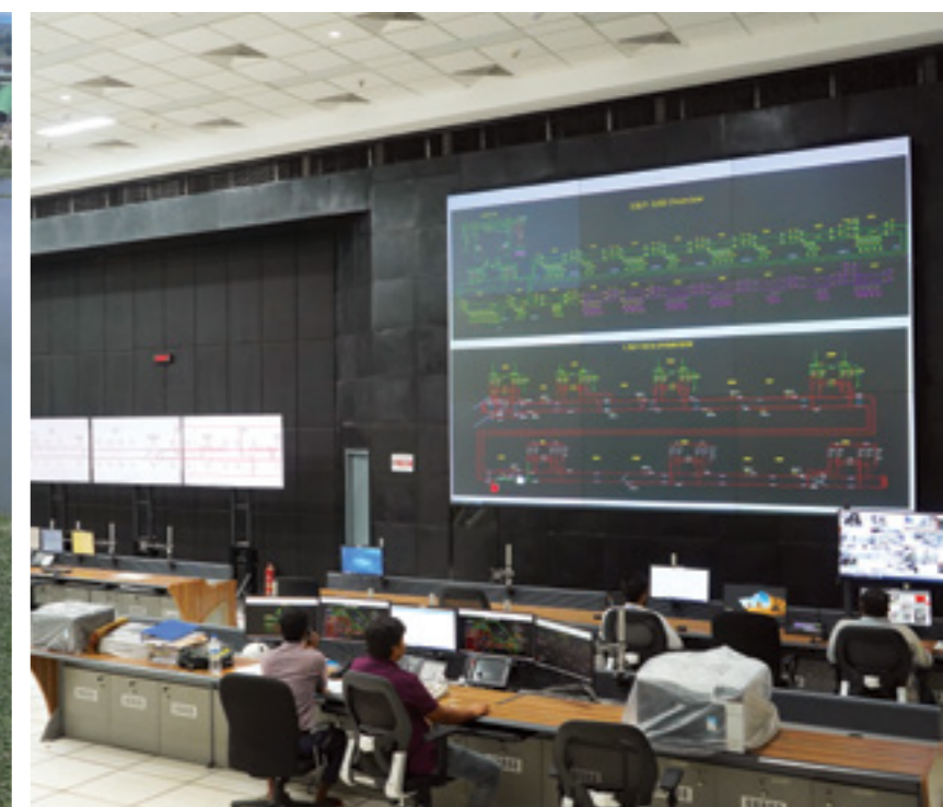
State of the Art - Operations Control Centre
