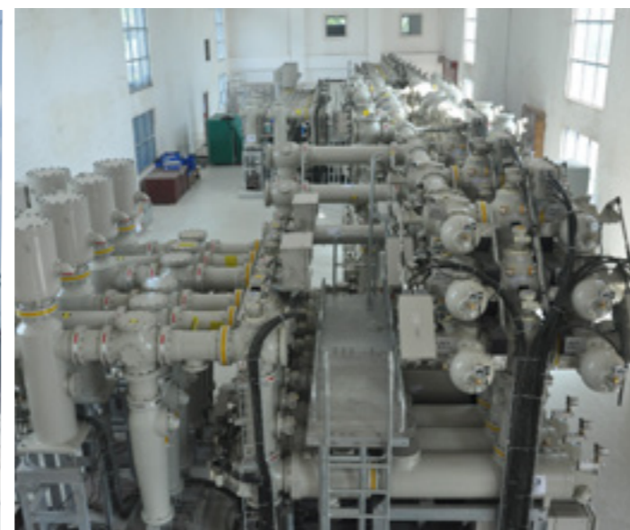
Gas Insulated Switchgear at Kharbao, WDFC
