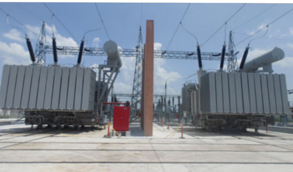
Scott Transformer in WDFC
