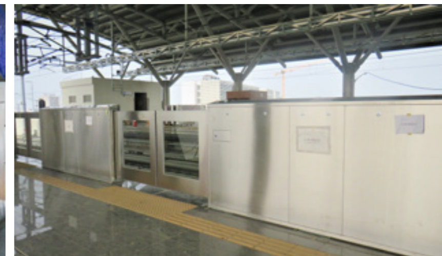
Platform Screen Doors
