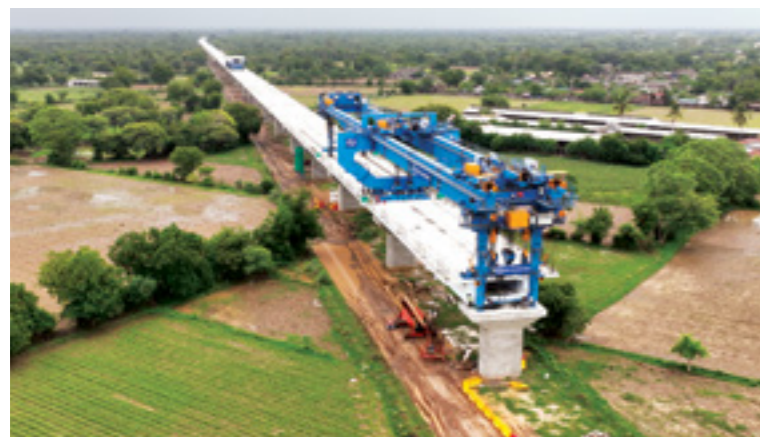
Viaduct construction in MAHSR - Full Span Girders weighing around 980 MT being launched using Launching Gantry
