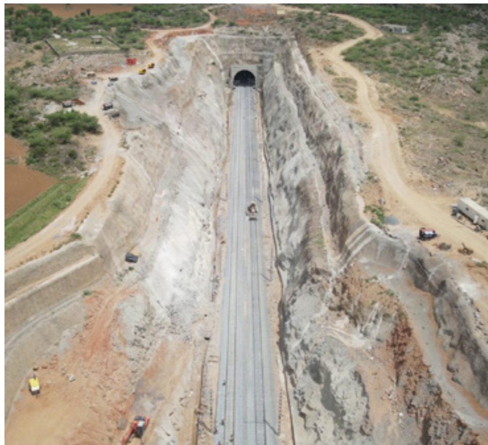
14m dia (Double Track, High Rise OHE) Railway Tunnel through Drill & Blast method in Aravalli Hills with large scale deep cut section to Tunnel approach - WDFC CTP 14 Project
