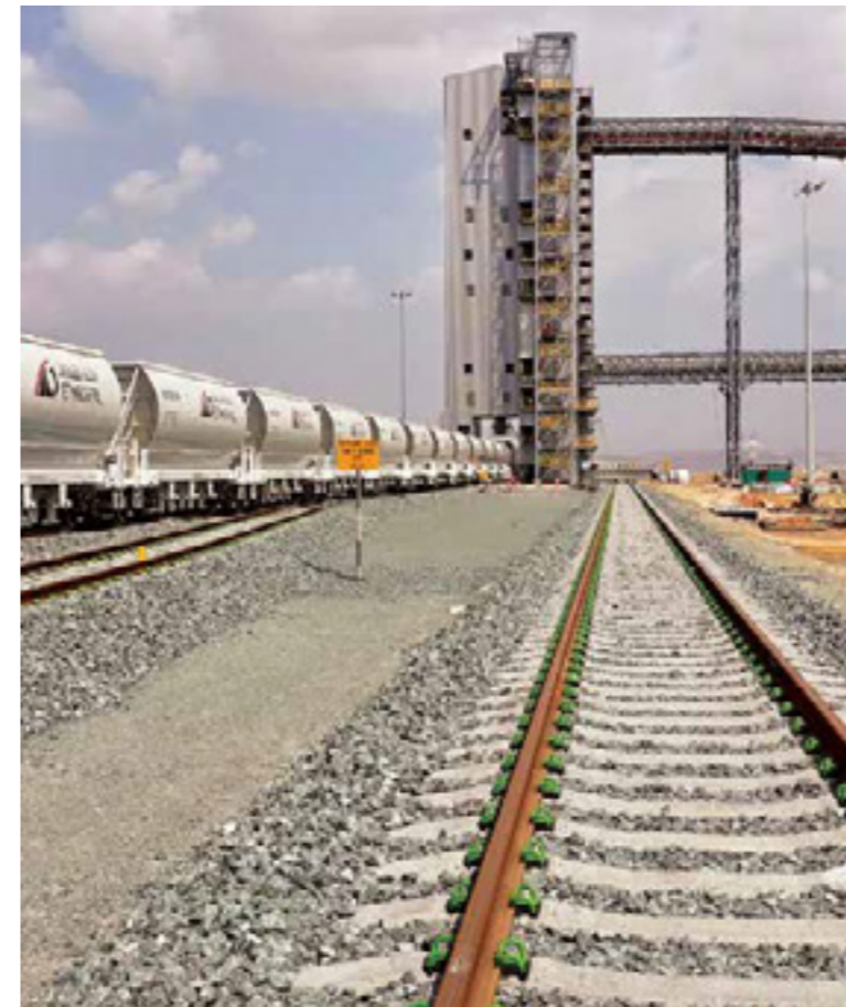
Freight Terminal in the Industrial City of Abu Dhabi (ICAD), spanning over 2.7 million square feet - the largest inland freight railway terminal in UAE Railway Network.
