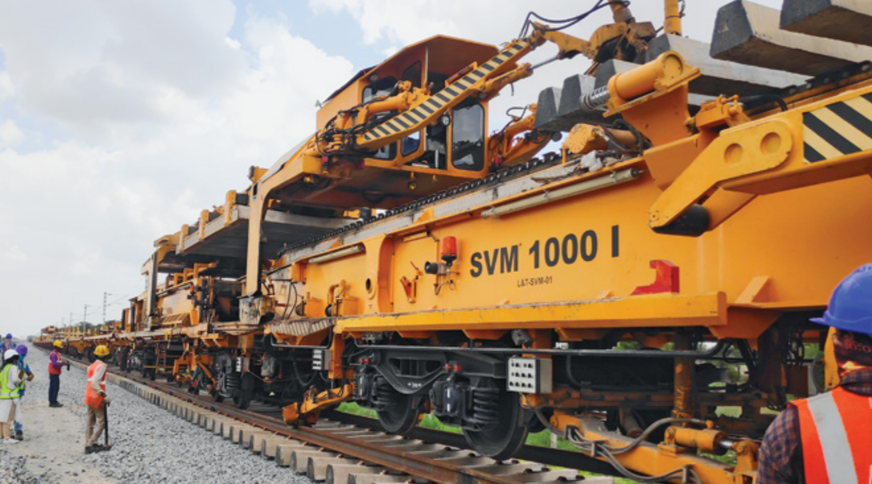
Plasser SVM 1000 at CTP 3R project - Mechanized methods for track linking results in high quality and speedy execution.
