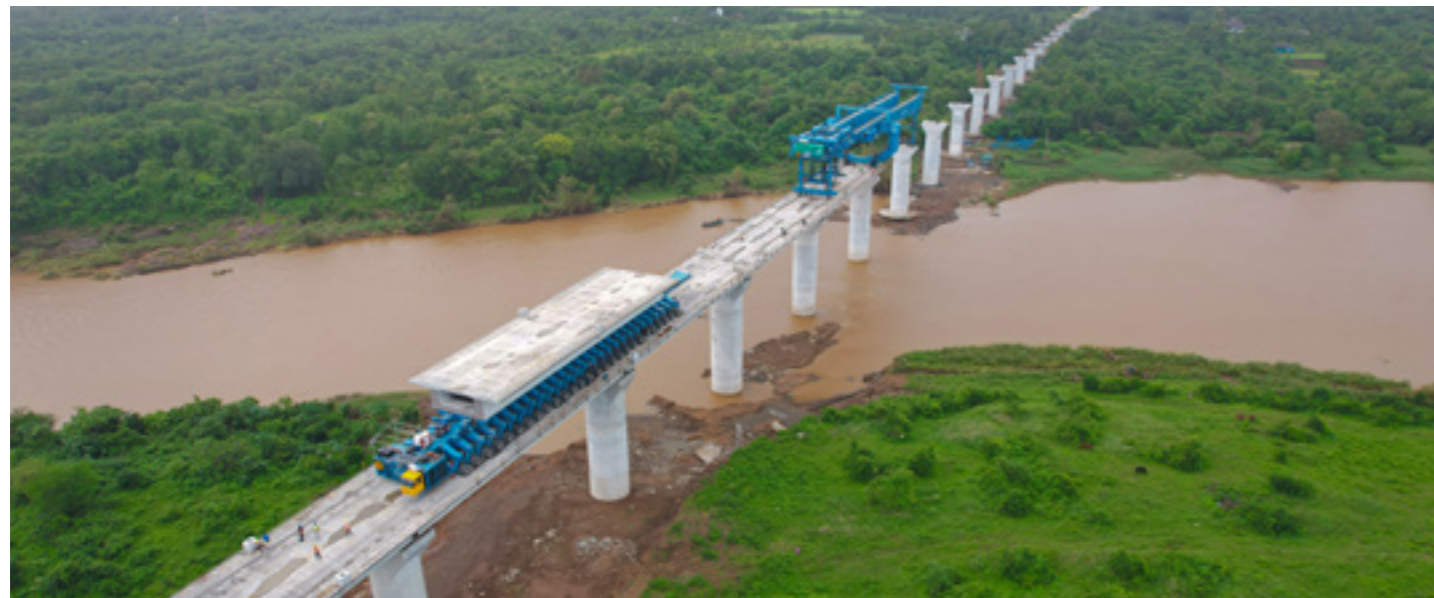
Viaduct construction in Mumbai Ahmedabad High Speed Rail (Viaduct Pkg C4 237.1km) - Full Span Girders weighing around 980 MT being launched using Launching Gantry
