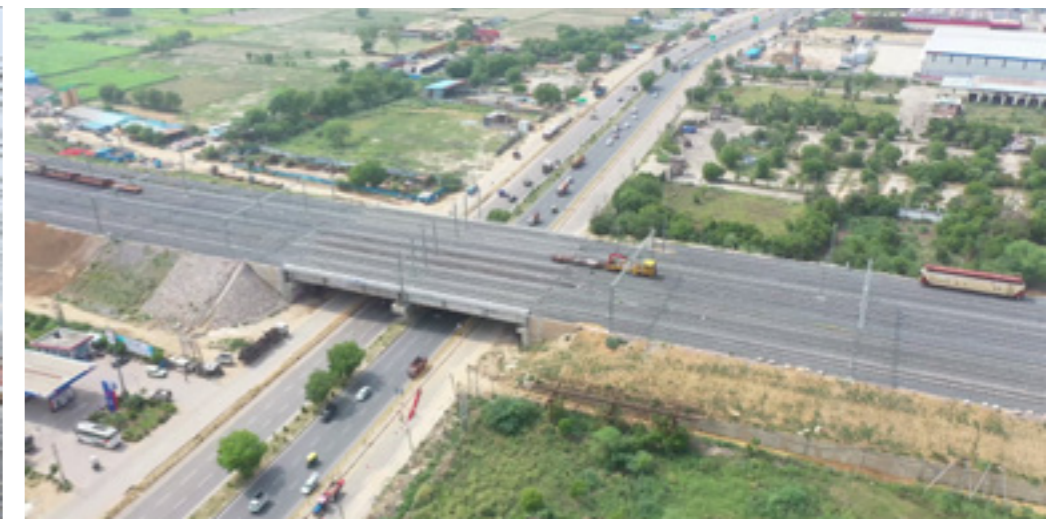
CP303 (Civil & Track) and CP 305 (Electrification and Signalling) - Khurja to Pilkhani 225 rkm
