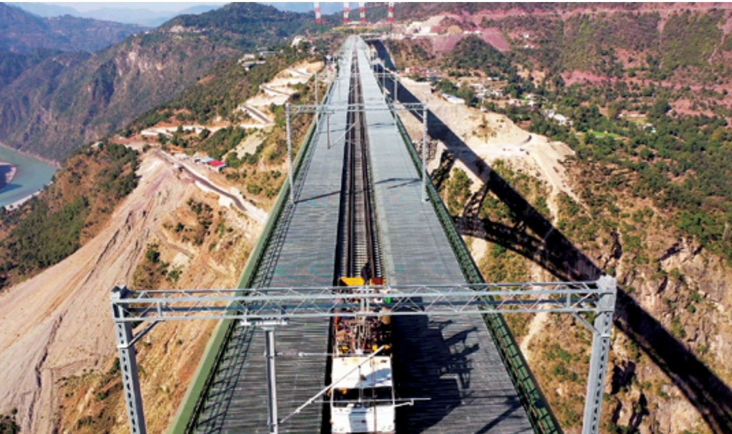
Electrification in Katra - Dharam sections in Jammu – Baramulla Railway including 19 tunnels, 84 Girder bridges and the iconic Chenab and Anjikhad bridges
