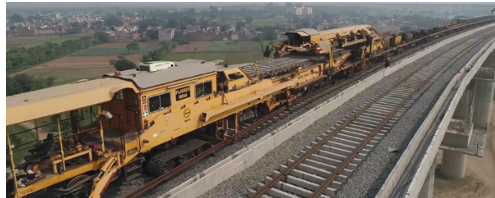
NTC at WDFC (CTP 14) - Mechanised Methods for Track linking results in High Quality and Speedy Execution
