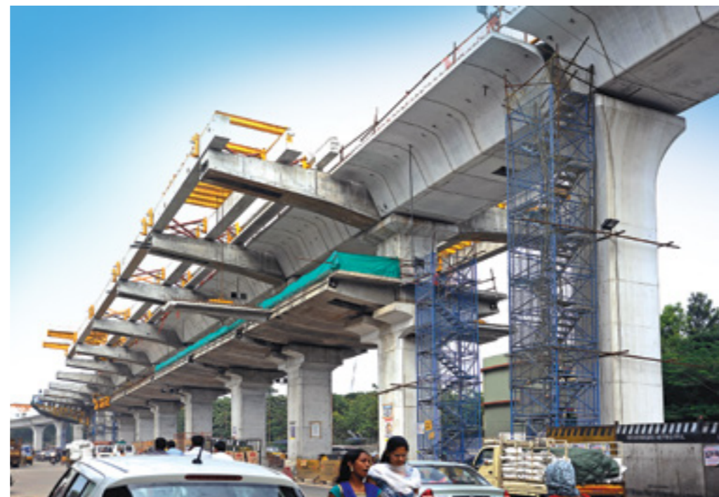
Concourse and platforms levels constructed entirely from pre-cast sections for Hyderabad Metro stations
