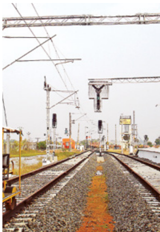
Open Training Yard for Track Laying, Railway Electrification and Signalling & Telecom at CDC
