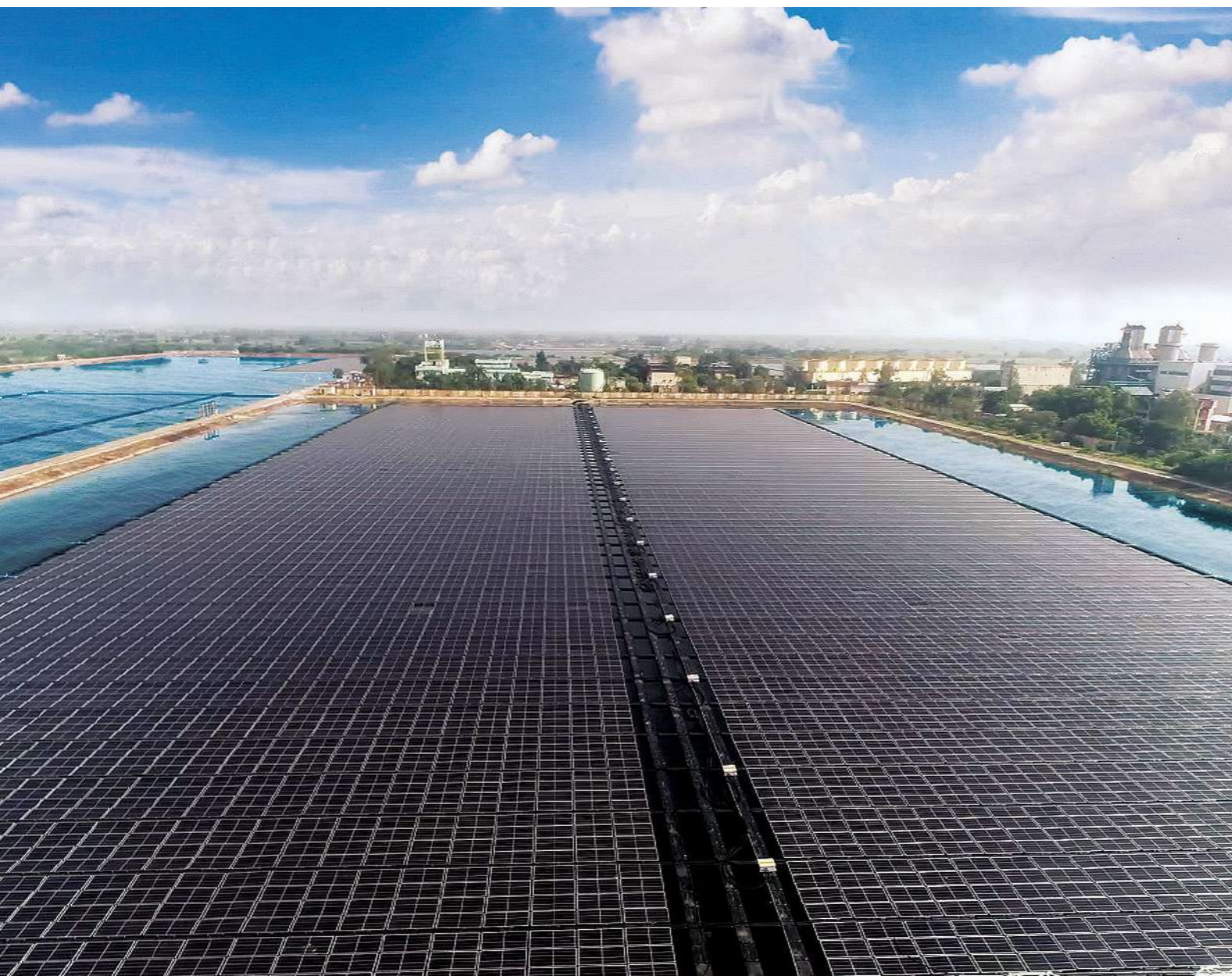
28 MWp Floating Solar PV Project in Auraiya, Uttar Pradesh
