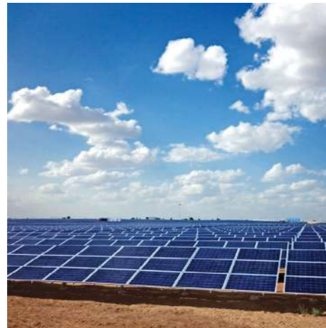
Crystalline - Si module technology based grid connected PV
