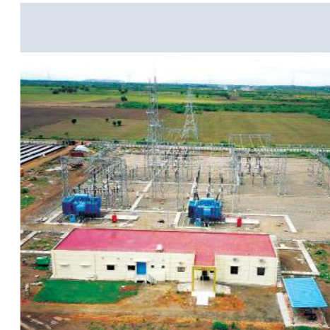
HV Substation and Transmission
