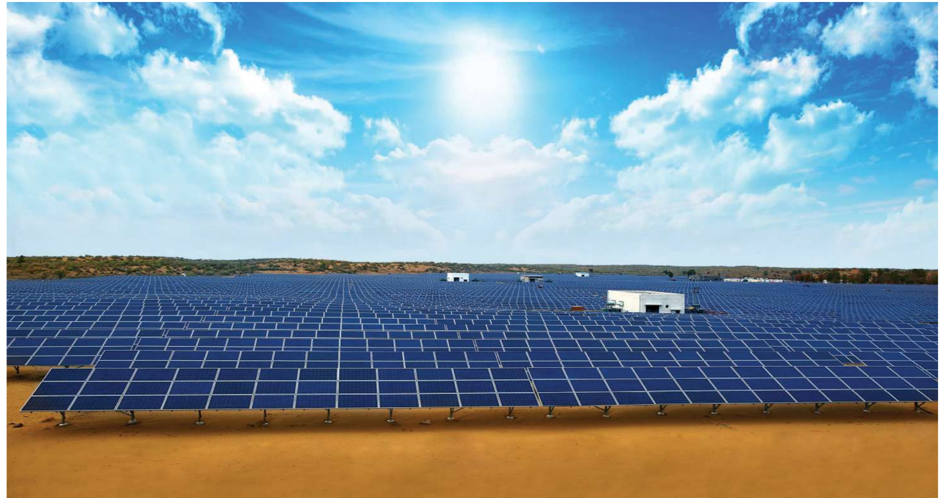
22 MWp Solar PV Power Plant at Rajasthan
