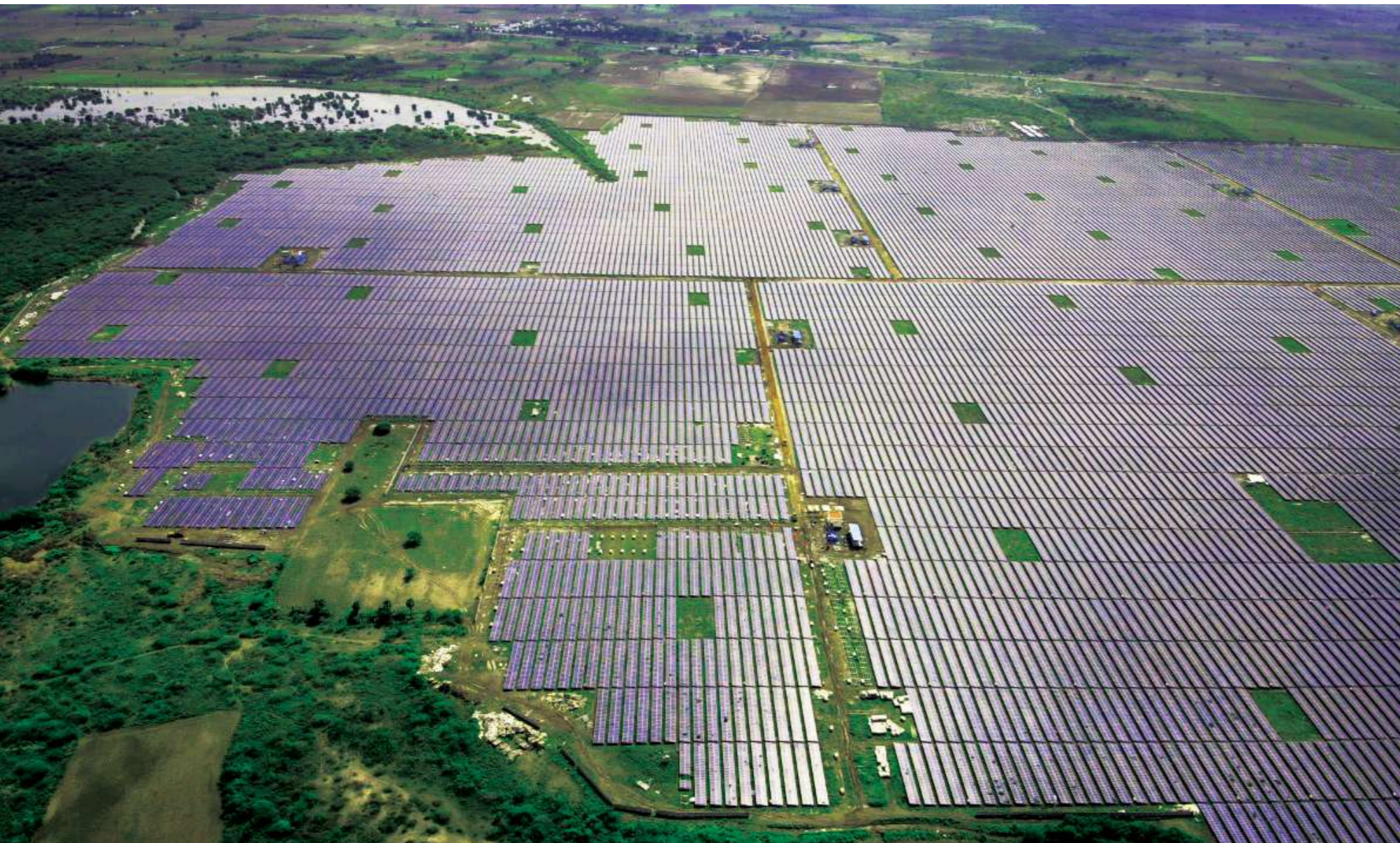
345 MWp Solar PV Project in Tamil Nadu
