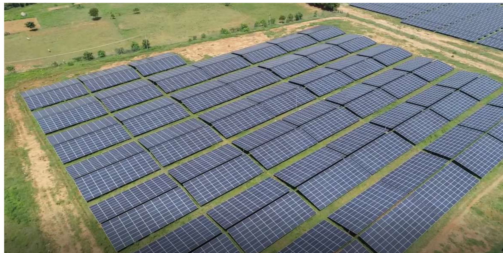
2.5 MWp East-West Solar PV Plant
