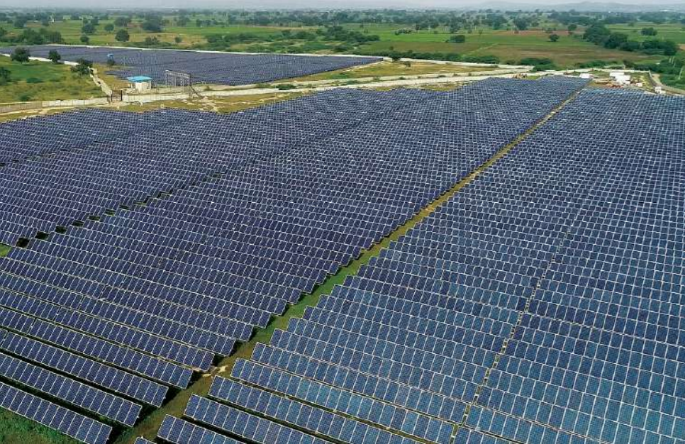
209 MWp/190 MW Solar Tracker Project, Karnataka
