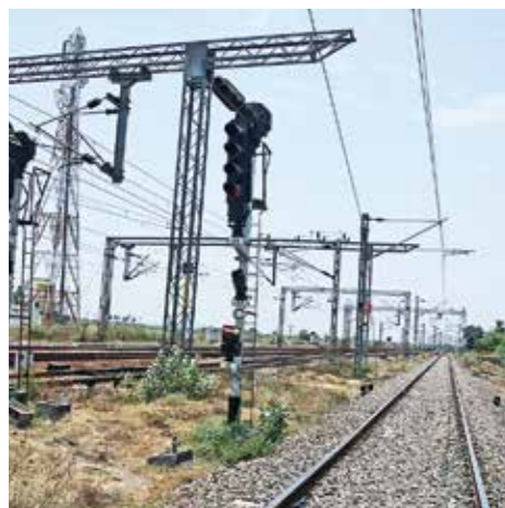
Signaling and telecommunication
