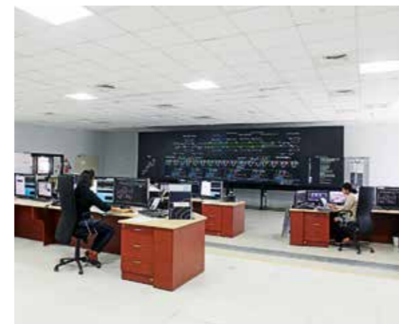
Operations and command centre of Mumbai Monorail
