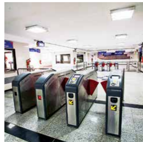
Automatic ticketing system at Mumbai Monorail
