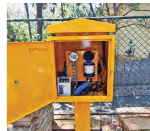
District meter cabinet
