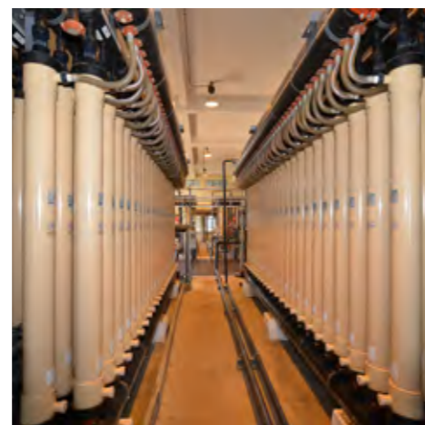
Asia's largest Micro-Filtration Plant of 158 MLD at Raichur, Karnataka
