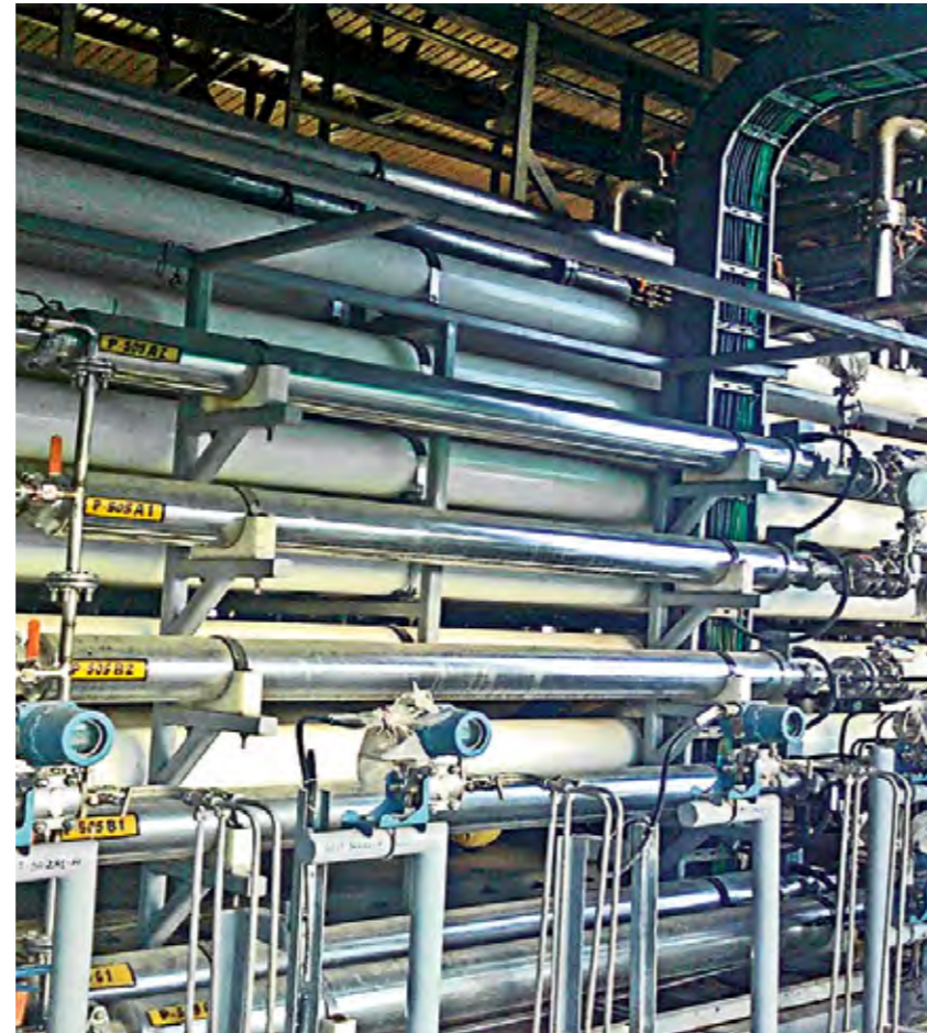
Reverse osmosis technology at a desalination project
