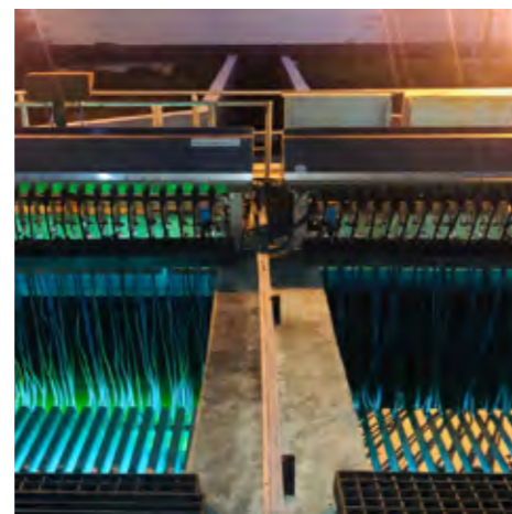
UV Disinfection System
