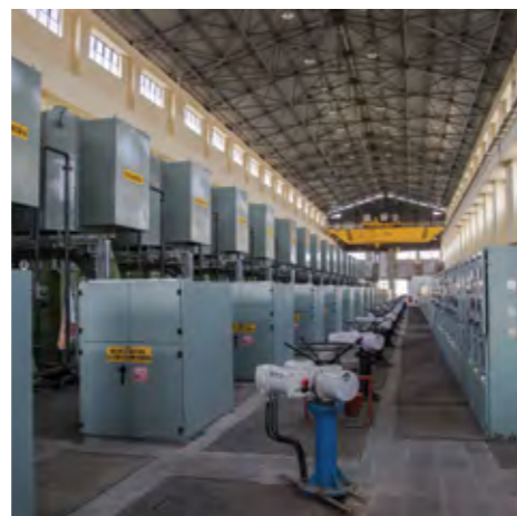
Pump house at Hanamapur, Karnataka
