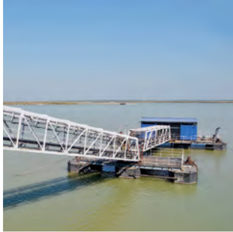
Floating barge intake, Sahibganj, Jharkhand
