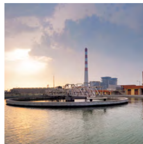
Plant Water System, Sagardighi, West Bengal
