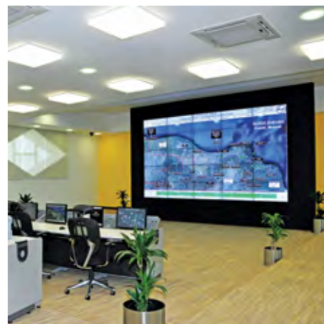
Real-time Project monitoring with SCADA
