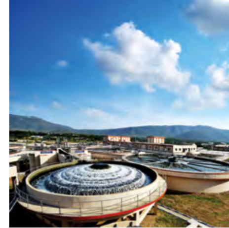
181 MLD Water Treatment Plant, Vellore, Tamil Nadu
