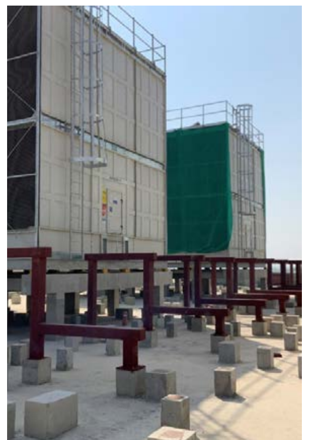
Cooling tower at the Club House
